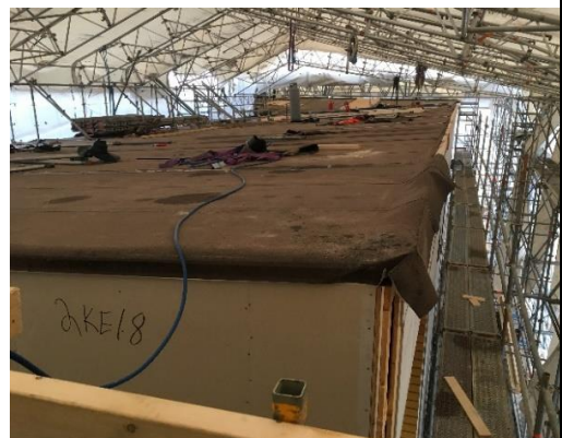
Two more floors of wooden large elements were installed under the tent for a 100 years old downtown block in Tampere.
