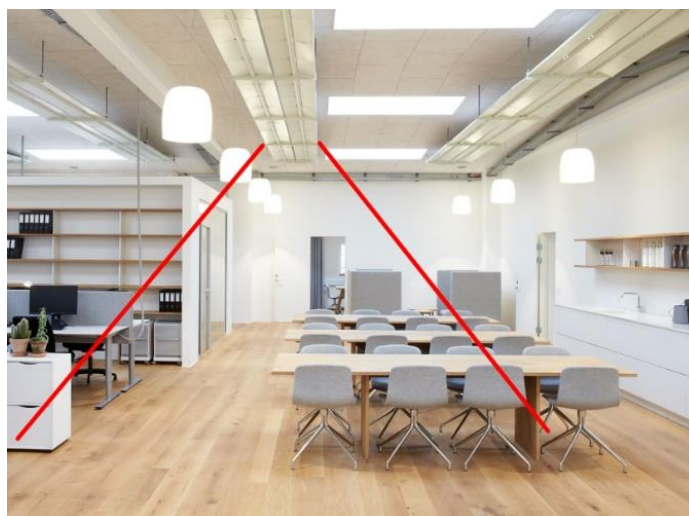
Fig. 3.43. Radiators placed in the ceiling.
