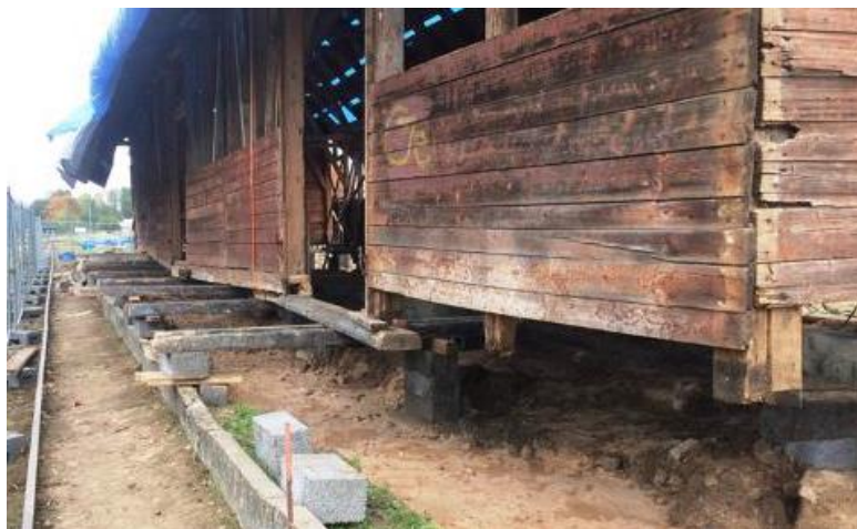
Fig. 7.10. Wooden stands, planking before rebuilding (Gadalabākābūve Latvijā 2018, 2019. The best building of the year in Latvia, 2019).
