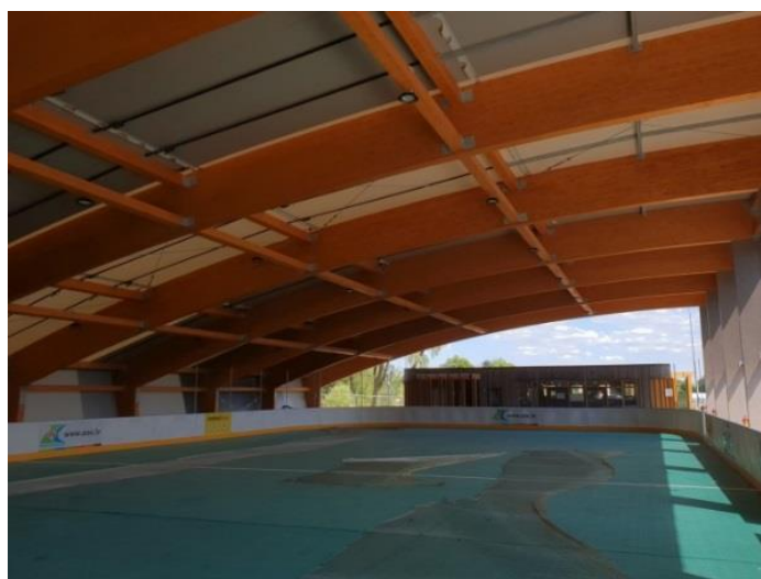
Fig. 7.13. Inside view (final view) (Gadalabākābūve Latvijā 2018, 2019. The best building of the year in Latvia, 2019).
