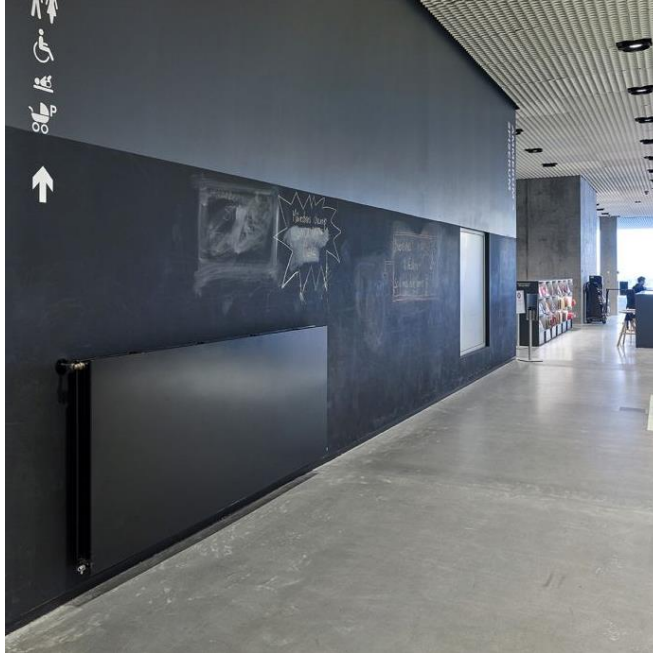
Fig. 3.46. Radiator outside the wall (Hudevad, 2019b).
