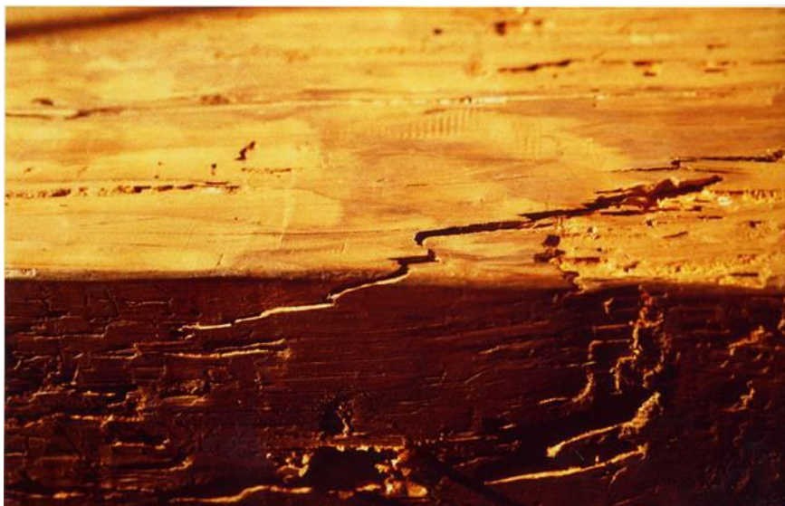
Fig.6.37. Beam cracked by bending. The crack extends from the sides to the bottom edge (Tampone, 2007).
