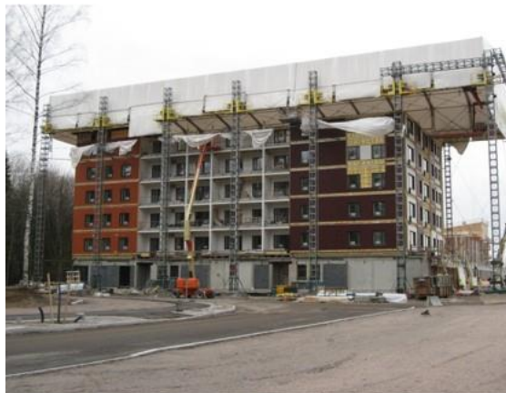
This project was a six-storey prefabricated large timber element project for housing fairs in Vantaa, Kivistö 2016. Total floor area of the project was more than 10 000 sqm. including about 200 apartments. The project was built by Rakennusliike Reponen Oy. Pftos: Rakennusliike Reponen Oy 2016.
